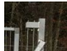
View of cable connection to welded bracket
