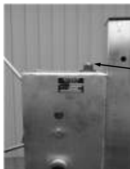
Close up view of cable connection on top of winch
