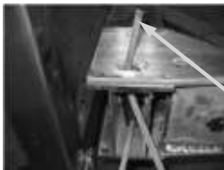
Winch column view of twin beam and front to back member together.
