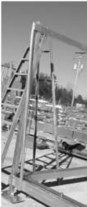
Front of hoist non winch side
